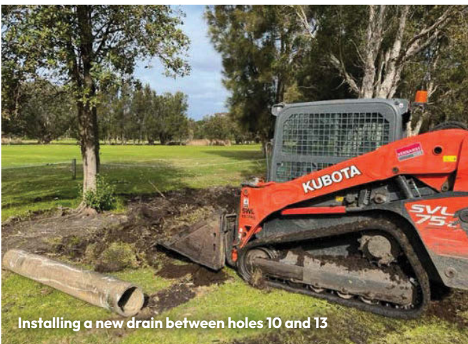
Team member John D working on the drain next to the 3rd hole
